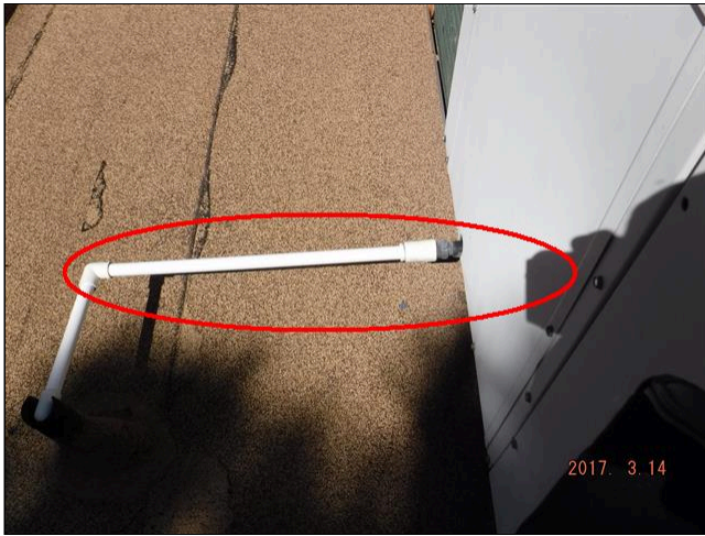
11.3 CONDENSATE PROVISIONS (Picture 1)
