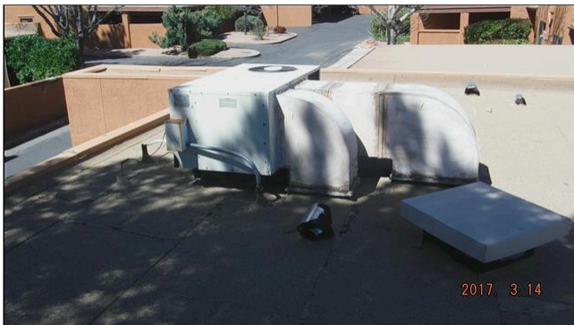
11.1 OUTDOOR UNIT WITH SAFETY SHUT OFFS (Picture 1)
