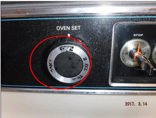
7.4 RANGE (Picture 2) Worn controls
