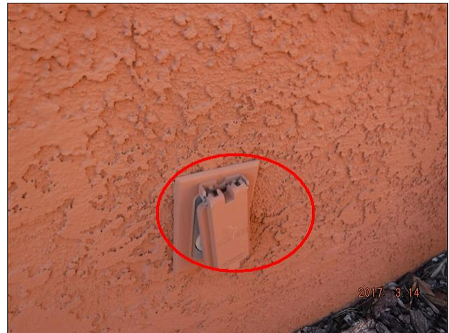
2.7 ELECTRIC / GFCI (Picture 1)
