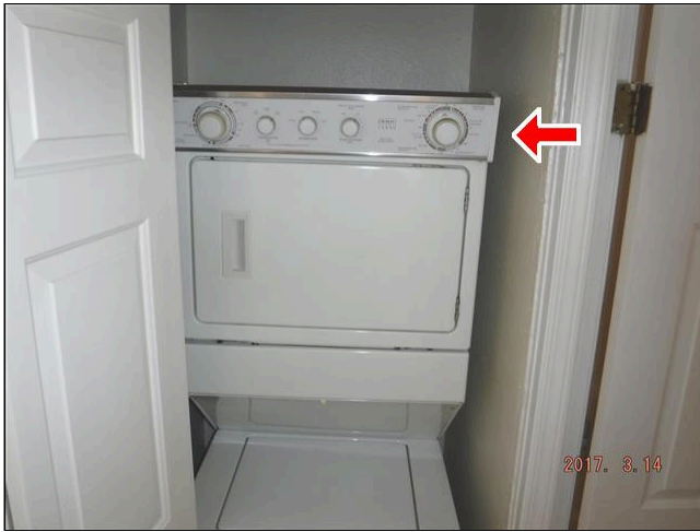
13.5 LAUNDRY AREA AND VENT FAN and dryer vent (Picture 1)
