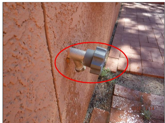
13.4 EXTERIOR FAUCET(S) (Picture 1)
