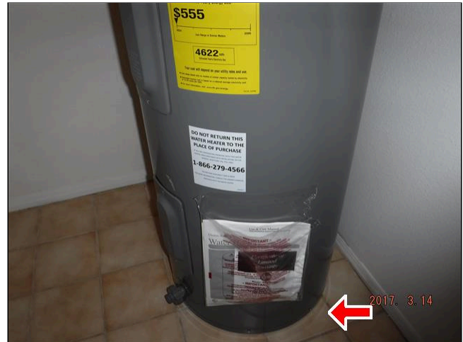
14.0 WATER HEATER SYSTEM 1 (Picture 2)
