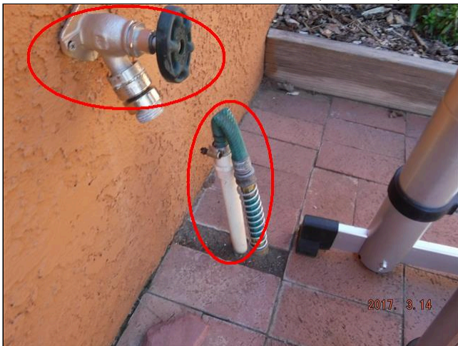
2.8 EXTERIOR FAUCET(S) (Picture 1) Possible landscape water hose
