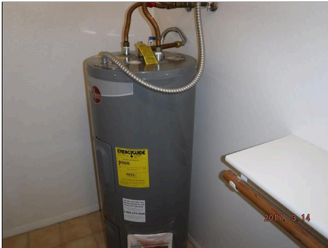
14.0 WATER HEATER SYSTEM 1 (Picture 1)
