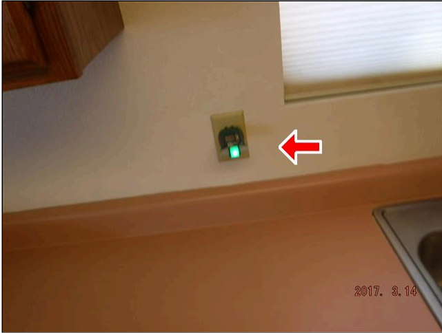
7.3 ELECTRIC / GFCI (Picture 1)
