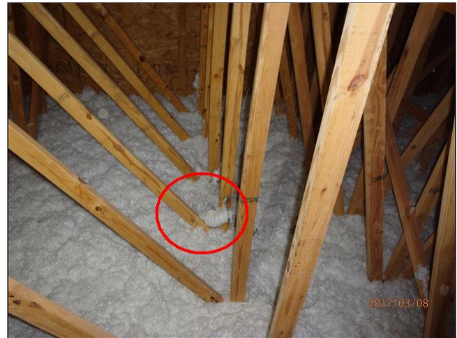
2.4 VENTILATOR DISCHARGE (.1) Item 2(Picture)
