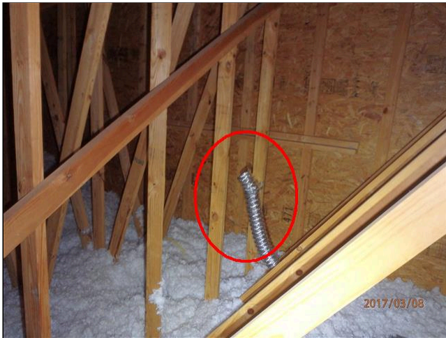
2.4 VENTILATOR DISCHARGE (.1) Item 1(Picture)
